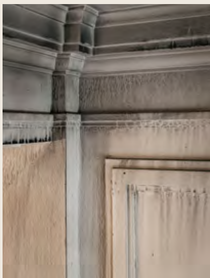
Smoke, soot and water damage on the internal walls of the building. Photo: Lean Timms
